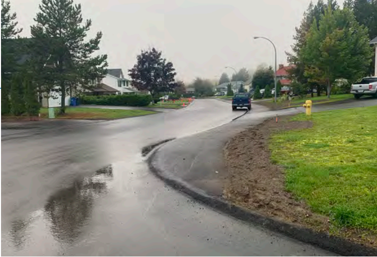
Left: In 2020, Public Works crews completed road reconstruction in the 5200 block of Mountain Vista Road.
