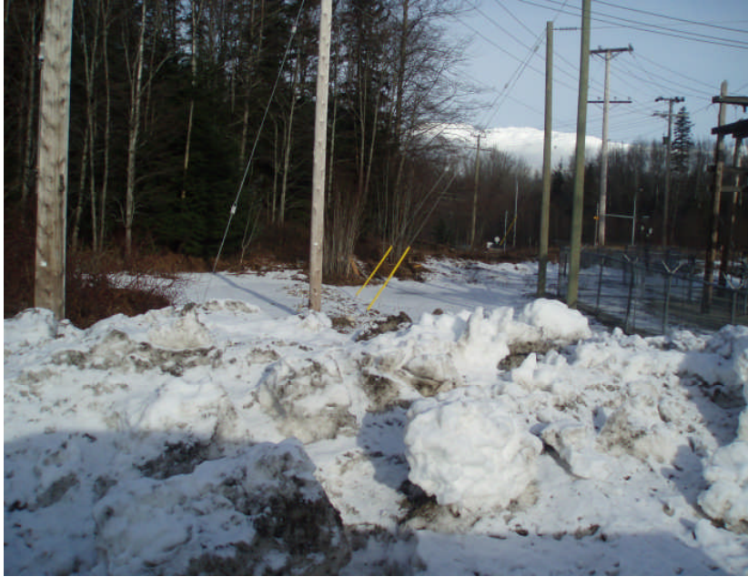
Forest fuels directly adjacent to BC Hydro sub station at 4- way intersection in Thornhill. Substation is constructed of large dry timbers.
