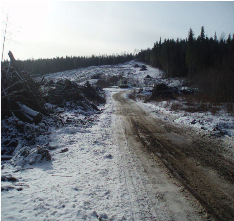
Example of private land clearing with no hazard abatement. This parcel of land is surrounded by low density development with some houses located directly uphill of this site
