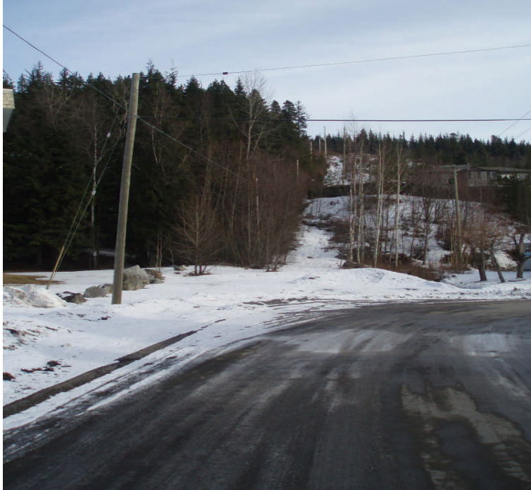
Hydro Line that provides power to City of Terrace water reservoir at the east end of Halliwell Avenue.
