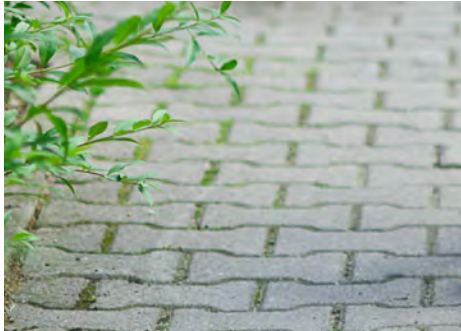
Streetscape designs should utilize durable materials - including hardscape and landscape elements - that are easily maintained
